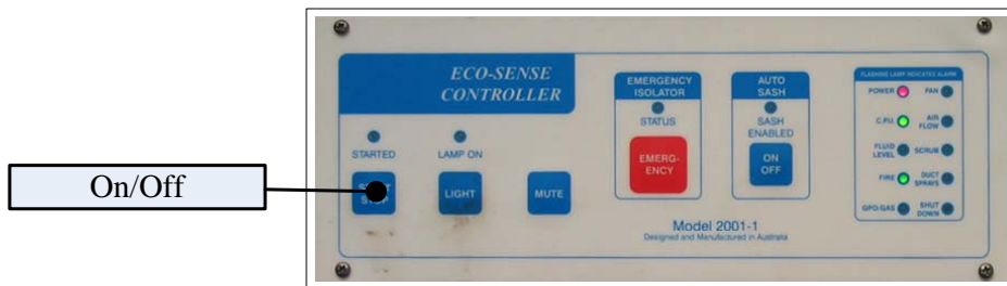
Figure B.4: Close up of control panel
